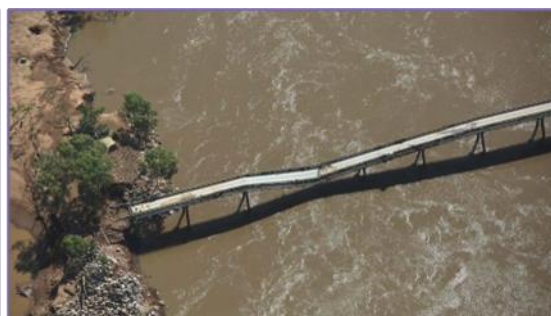
Image 2: Damaged Bridge into Fitzroy Crossing 2
